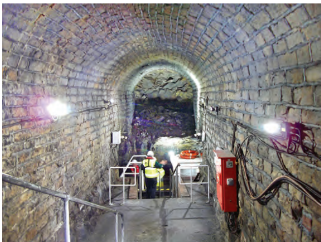
The safety adit, looking back at the canal, showing the boat used by Sub Brit to traverse the tunnel. Photo Adrian Armishaw
